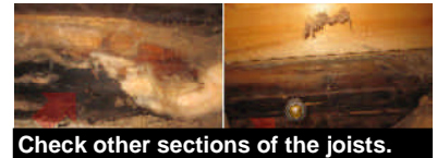
Check other sections of the joists.
