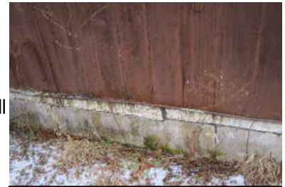
Concrete not visible, cover insulation.
