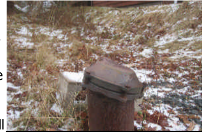
Install cap properly, protect from vehicle
